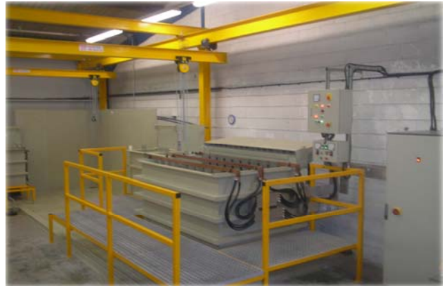
Pickling & Electropolishing Plant
